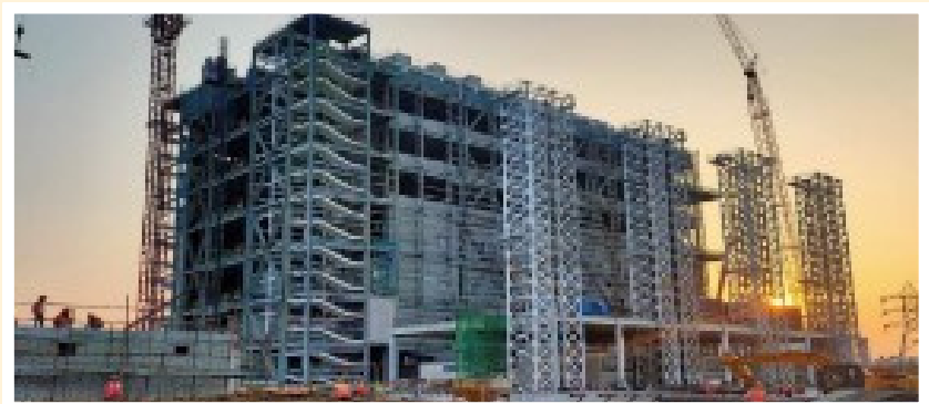
Fig 23 : AdaniConneX Centre, Chennai
